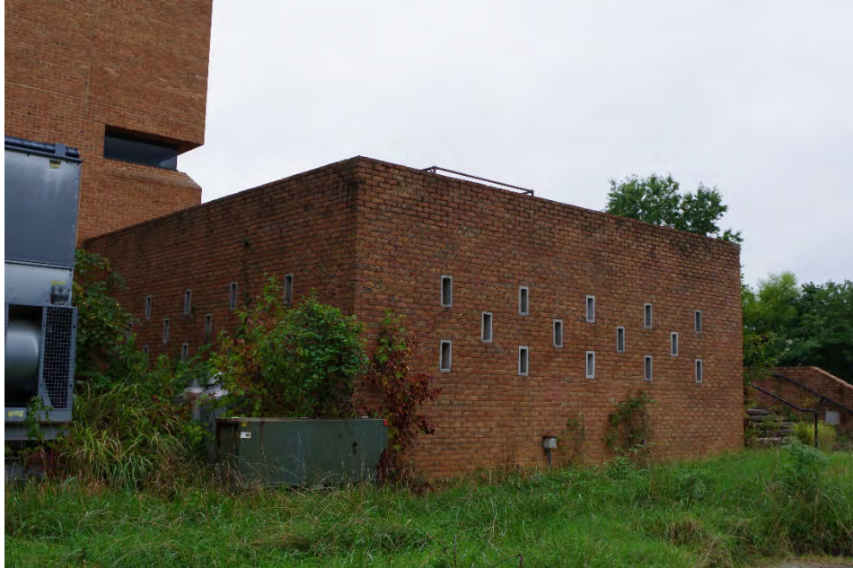
Photo 17 of 47: Brick Wall Shielding Utility Machinery on the Northwestern Façade, camera facing south.
