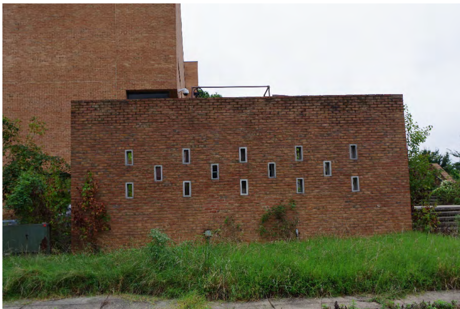
Photo 18 of 47: Brick Wall Shielding Utility Machinery on the Northwestern Façade, camera facing southeast.
