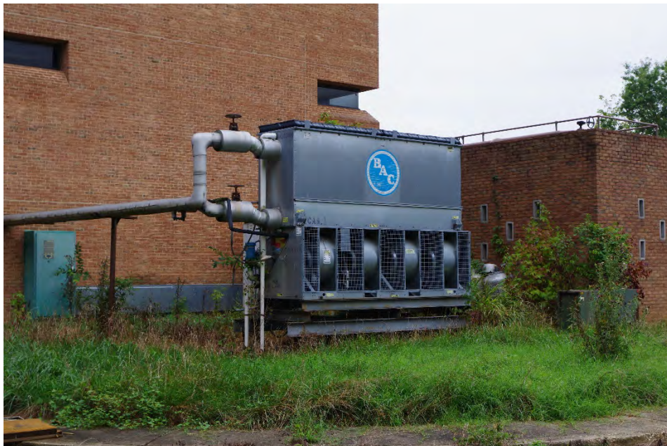
Photo 16 of 47: View of Air Conditioning Unit on Northwestern Façade, camera facing south.
